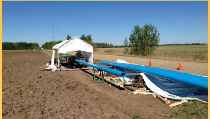
Residents will see much the same above-ground activity as they did during the installation of the pipeline from the Bonanza water treatment plant into the center of Bonanza.
