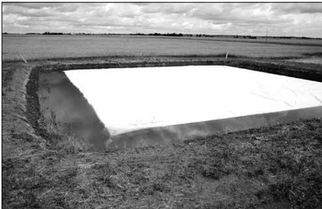
Figure 4. Plastic cover to reduce dugout evaporation losses
