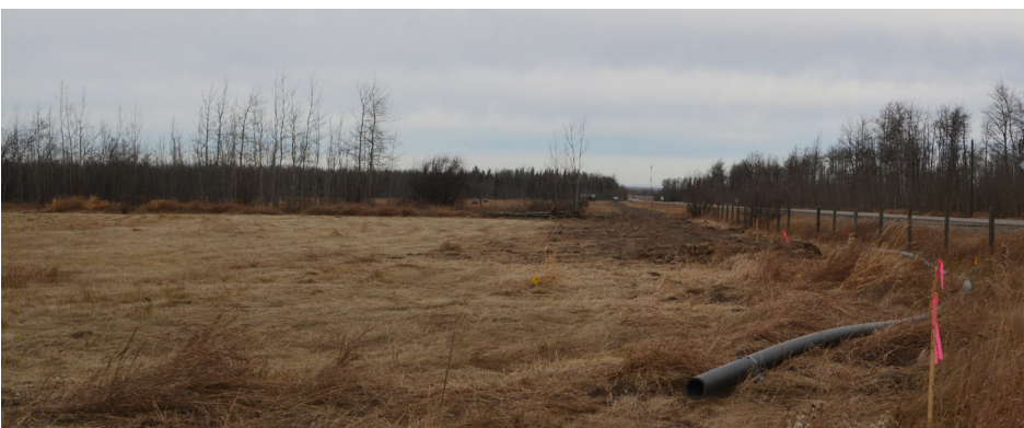
After the pipeline has been buried into the ground, Tri-line Contracting returns the land to as close to the way they found it as possible.
