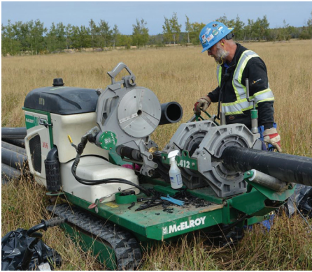
Lengths of pipe are cut, trimmed and fused together using specially designed equipment.
