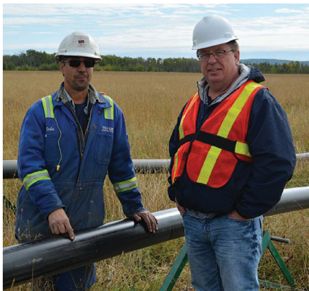
Dale Gour (left), owner of Tri-Line Contracting Services and Saddle Hills County Manager of Environmental Services Darren Lubeck (right) seen just south of Bonanza September 21, 2018 during the initial process of fusing main supply line for the Bonanza – Bay Tree main supply line.
