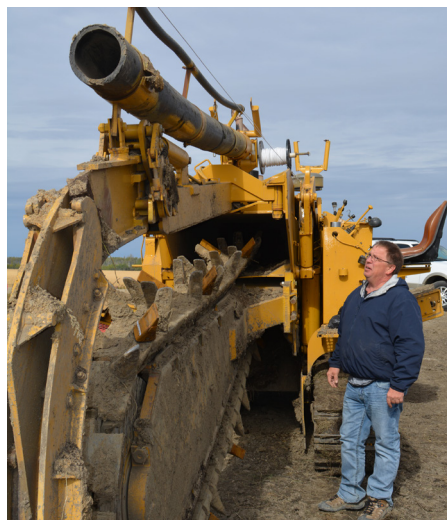
Saddle Hills County Manager of Environmental Services Darren Lubeck inspects one of the trenchers being used to dig a path and lay the pipeline as it moves across the land from Bonanza to Bay Tree.
