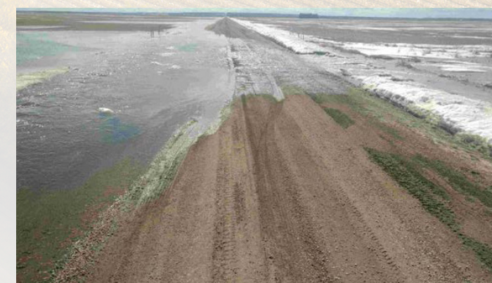
Ditch ‘Ice/Snow Dam’ creating flooding on fields and the road
