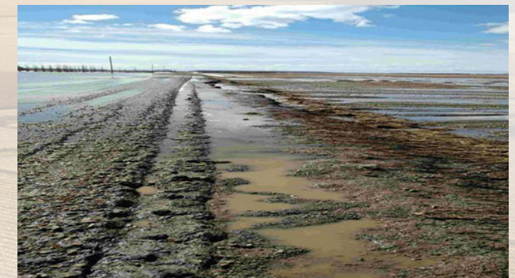
Road wash-out due to field flooding
